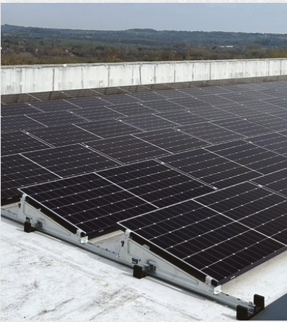
SOLAR PANELS ON ROOF
