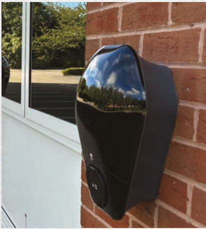
7kW EV chargers
